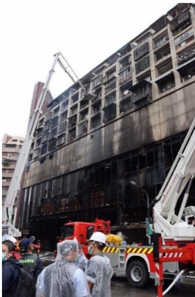
Cheng Chung Cheng Building after the fire.
